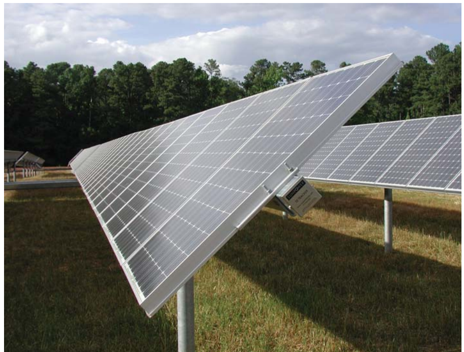
The SAS Solar farm solar panels.
